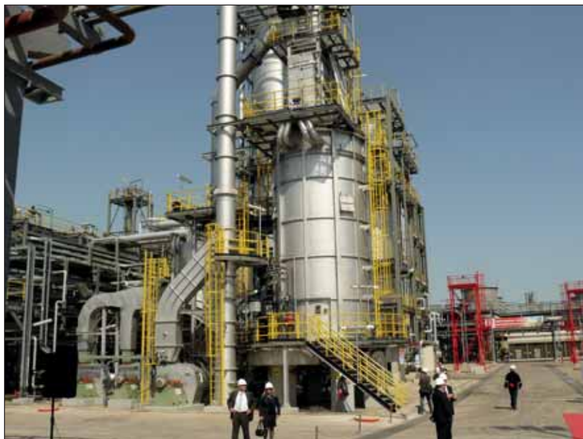
Installation at Lukoil – Neftochim near city of Burgas – the biggest petrol refinery in Bulgaria. According to Bulgarian National Television News, Lukoil produces around 80% of the fuels for the Bulgarian market.
